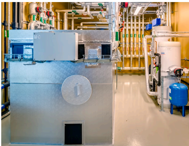
Fig. 3. The PPTES unit [32]. It is housed in a thermally insulated container.
