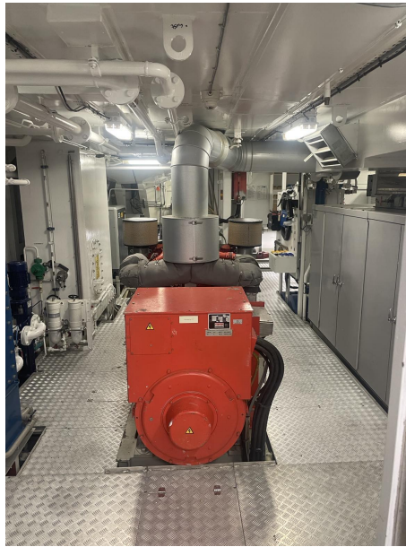
Figure 4.4: Port side of the engine room, showing one of the three diesel generators.
