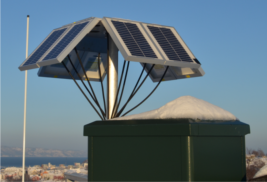
Figure F.41: Setup of the nine solar panels.
