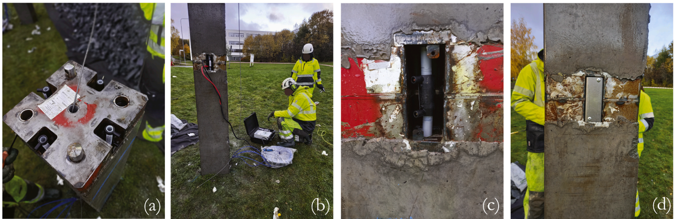
Fig. 8. Installation of DEPs in Trondheim using DEP Joint, (a) after the installation of the bottom segment, (b) coupling the pipes after the top segment is connected to the bottom segment, (c) the pipe fitting after coupling the top and bottom pipes, (d) installing the shielding plate over the sidewall channel and riveting it to the joint.
