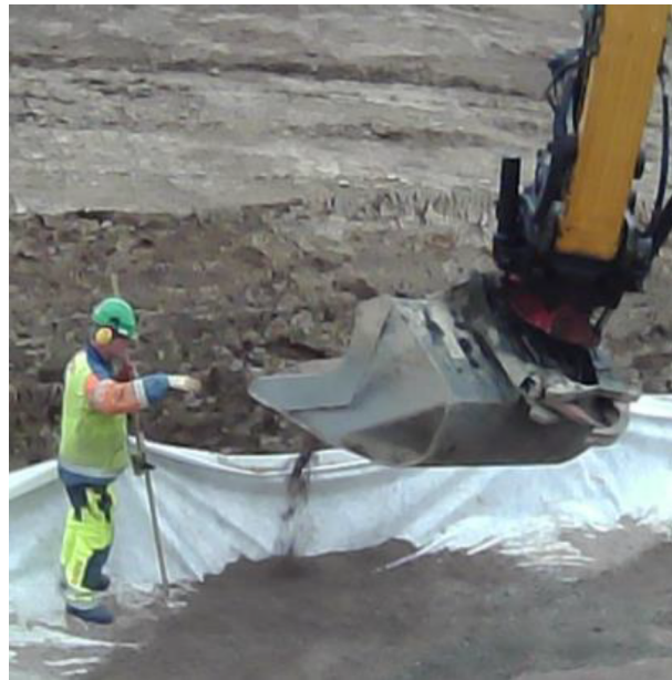
Fig. 1. The picture taken from the cabin of an excavator, which shows the ground worker giving instructions to the excavator operator about where and how much the gravel should be poured.
