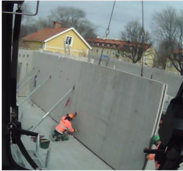
Fig. 2. The picture taken from the cabin of a mobile crane, which shows two ground workers ensuring the prefabricated wall panel is placed correctly.
