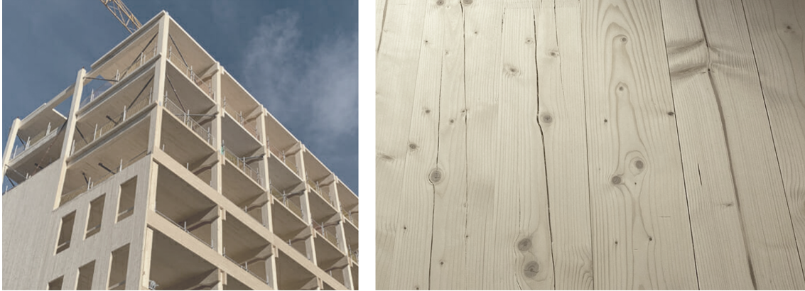
Figure 53: Spor X structure in CLT (left) and observed cracks in the cross-laminated timber (right)
