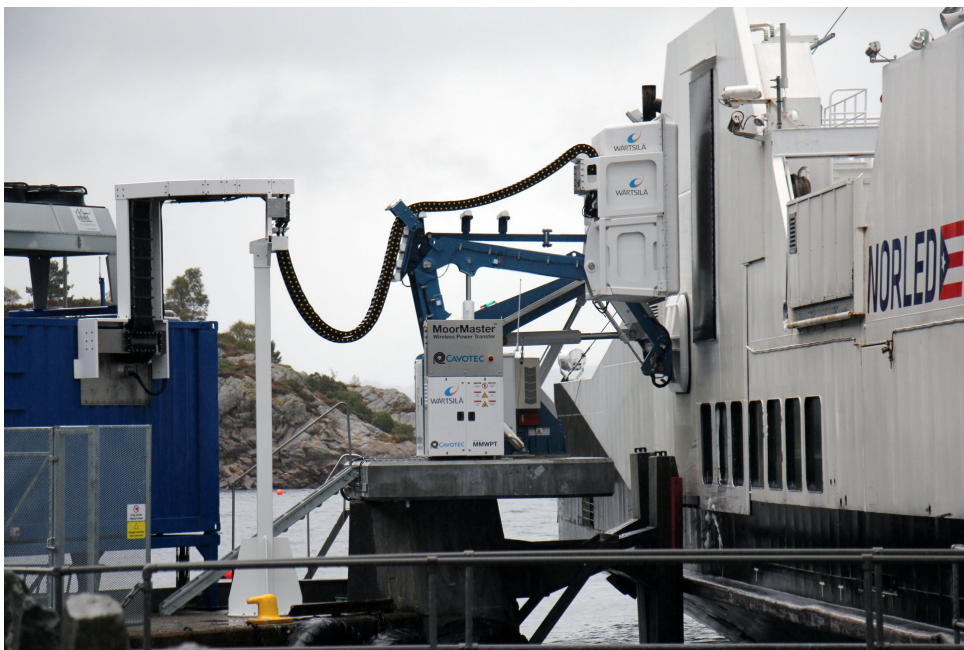
Figure 8.2: Cavotec MoorMaster and Wärtsilä's induction system in action on MF Folgefonn [81].
