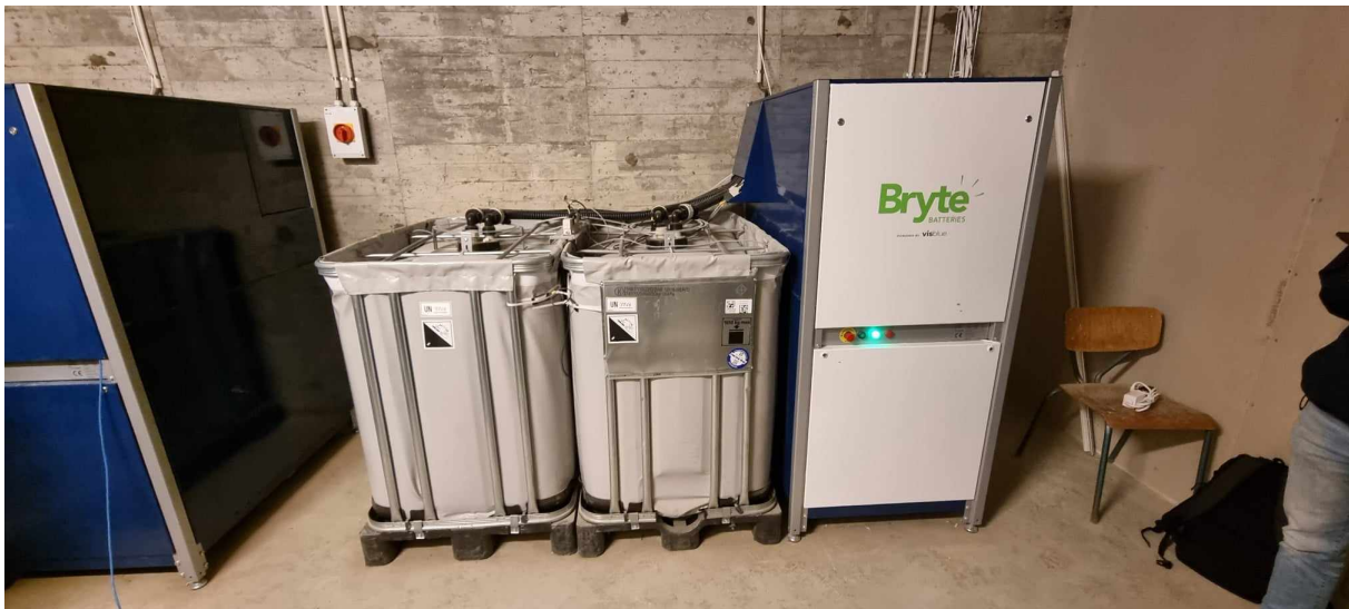
Figure 4.3: VRFB from Bryte Batteries.
