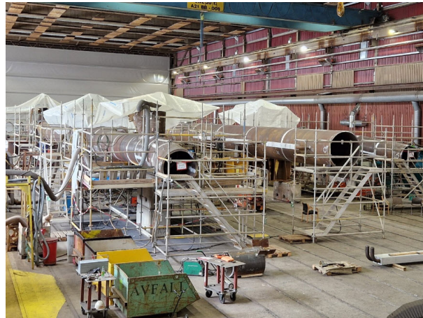
Figure 1: Current scaffolding setup in working hall A2 at Aker Solutions, with jackets lying horizontally.
