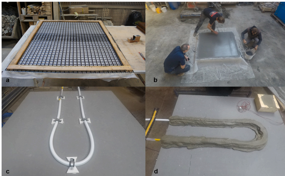
Fig. 4. Constructing the concrete panel. (a) Preparing the formwork and reinforcement for the lightweight concrete panel. (b) Placing and finishing the concrete layer. (c) Securing the TABS pipework to the concrete panel. (d) Applying the concrete cover to the TABS pipework and pipe surface temperature sensor.
