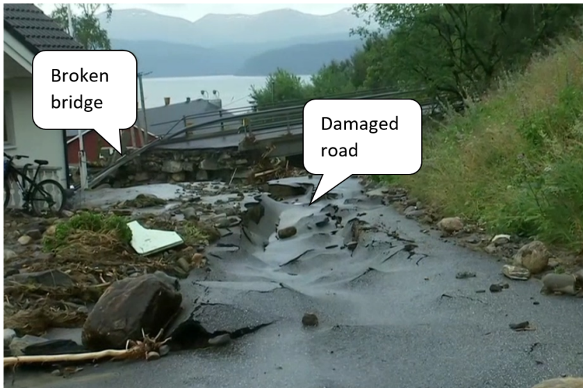
Figure 1.3: One of the damaged roads and bridge in the village. Source: tv2.no.
