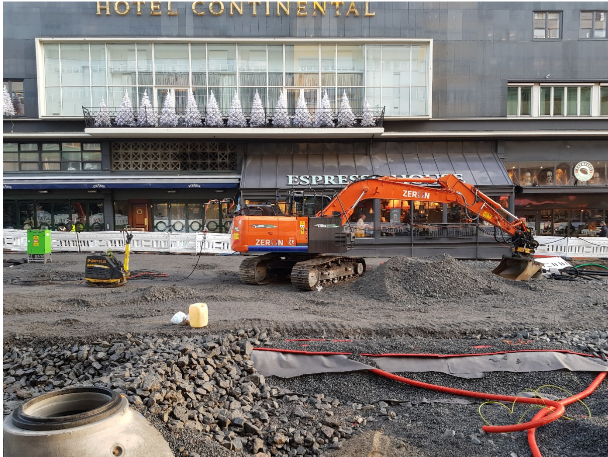
Figure 4 Photograph of the 17.5t excavator on-site at Olav Vs Street in Oslo, Norway. Source: SINTEF
