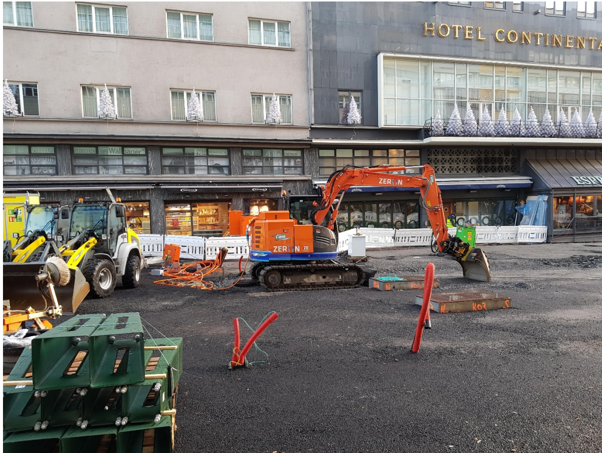
Figure 5 Photograph of the 8.5t excavator charging on-site at Olav Vs Street, Oslo, Norway. Source: SINTEF
