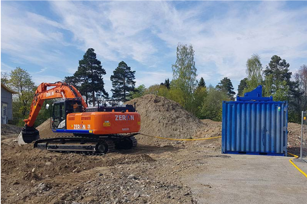
Figure 3 Photograph of the 38t excavator and cable container on-site at Biri care home in Gjøvik, Norway. Source: NASTA, used with permission
