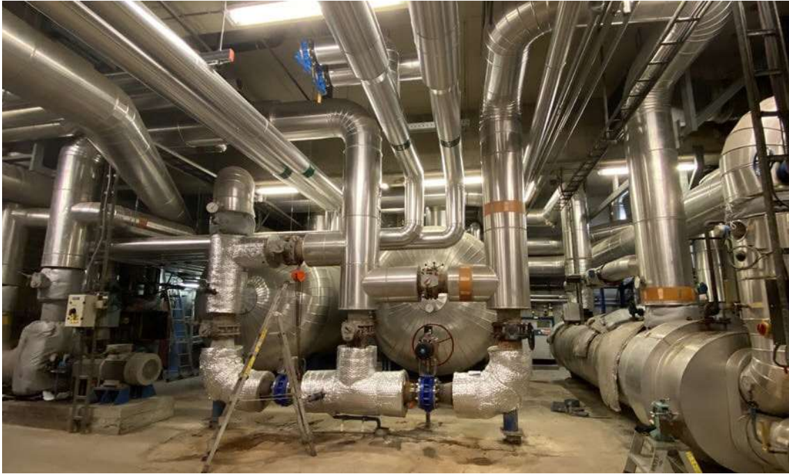
Figure 2-13: Boiler room for 3rd gen. DHN in Trondheim (Heimdal facility). Image Credit: Statkraftvarme.no [66].
