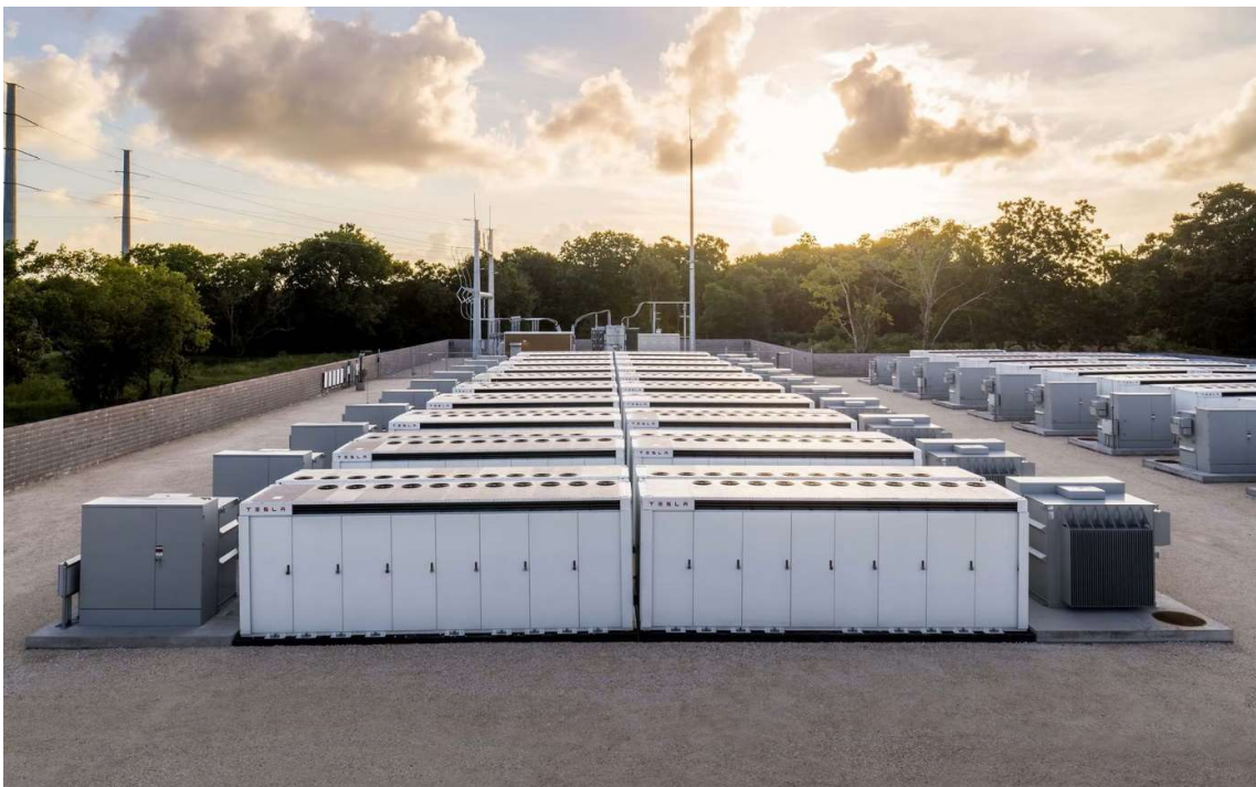
Figure 2-7: Tesla Megapack Grid Li-ion Battery in Western Australia. Image Credit: Tesla.com [41]
