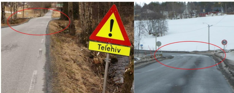
Figure 1 The damage to the road by frost heave. The left photo was taken at Vikevegen, from http://vikebygd.org . The right photo was taken at road FV26 in Norway, by Lars Andreas Solås.
