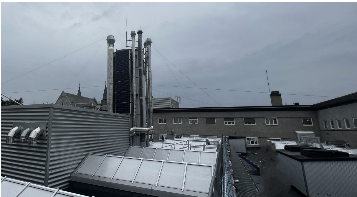
Figure 5.1: The PV panels on the roof of the Thermal Laboratory at Gløshaugen and a pyranometer mounted on a pole to the right in the figure.
