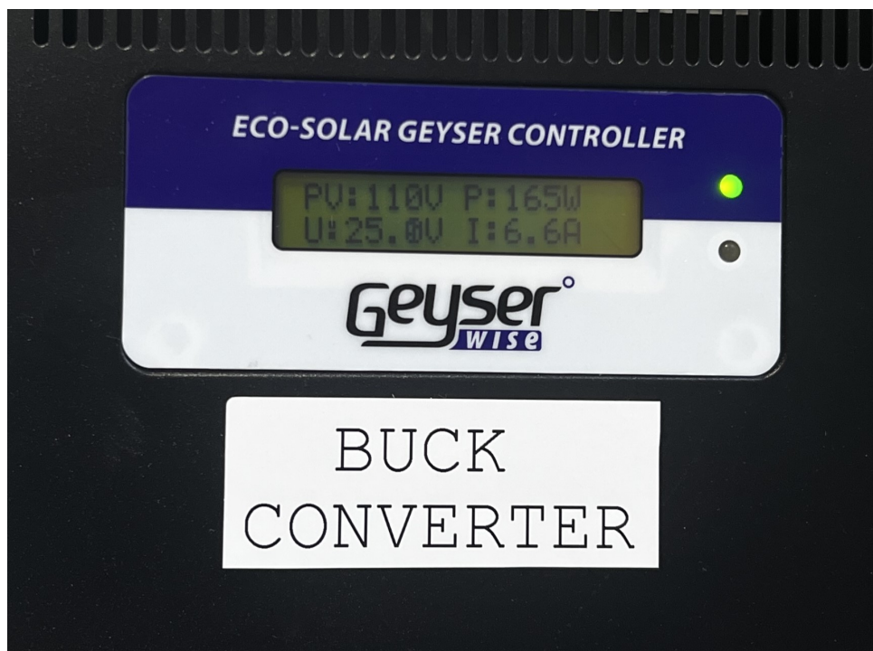
Figure 6.1: Readouts of the Geyserswise 72V controller. The display presents PV power in, with power, voltage and current out of the controller.
