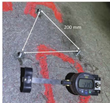
Figure 4. Procedure for direct measurements of shrinkage on the surface of sprayed concrete.
