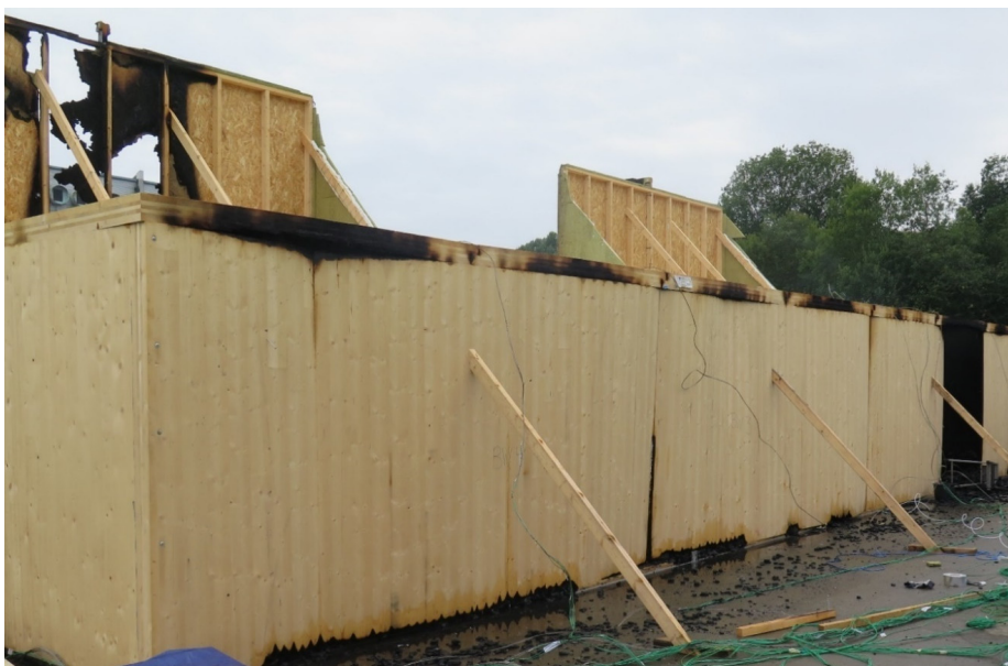
Fig. 45 Damages seen from the back side of the compartment of #FRIC-02 after the end of the experiment.
