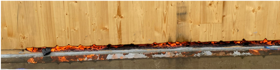
Fig. 29 The fire burned through the intersection between the back wall and the bottom plank at approximately 60 min. The image is taken at a later point when the gap had become larger. The lack of a fire sealant between the bottom plank and the CLT wall enabled this and highlights that connection details are crucial to fire safety.
