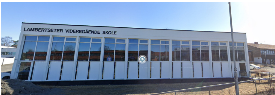
Fig. 71 The window wall of the school gym before the fire. The door to the left was blown open by the pressure. Photo: Google Maps/Google Street View.
