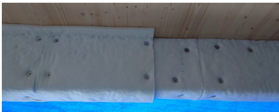
Fig. 49 The glulam beam was protected with two overlapping layers of 25 mm ceramic fibre insulation. This was sufficient to protect the beam in #FRIC-01.
