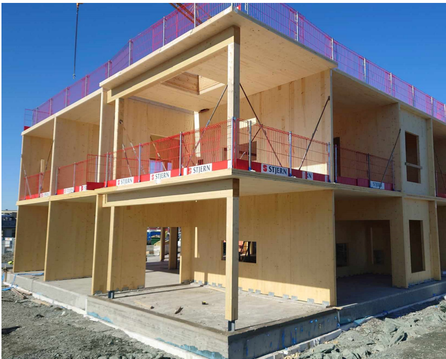
Fig. 1 Building under construction where load bearing CLT elements are used in walls and floors. Openings for windows and doors have been cut out during production.
