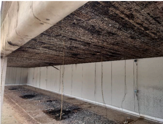
Fig. 14. Compartment after burn-out of the wood crib. No gypsum boards had fallen down, and the wood crib was completely consumed.
