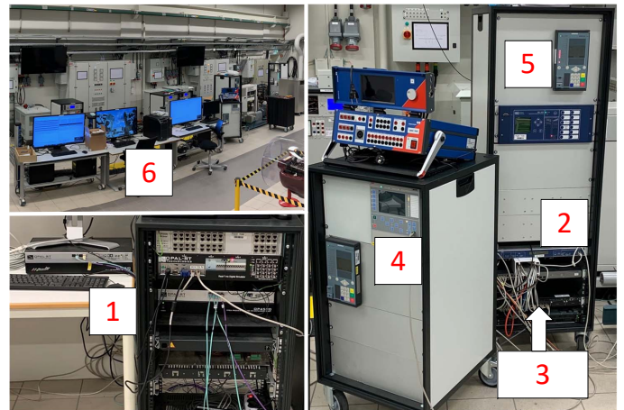
Fig. 2. View of laboratory and devices. 1: Real-time simulator, 2: GPS master clock, 3: power system substation communication switches, 4: PMU 2, 5: PMU 3, 6: Computers for PDC and Control centre DSE.
