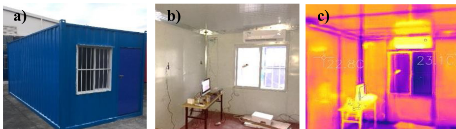
Fig. 3. a) Standard container building, b) Test of Vacuum Insulation Panels (VIP) with thermocouples and heat flow meters, c) Thermogram of the walls before the installation of VIP.
