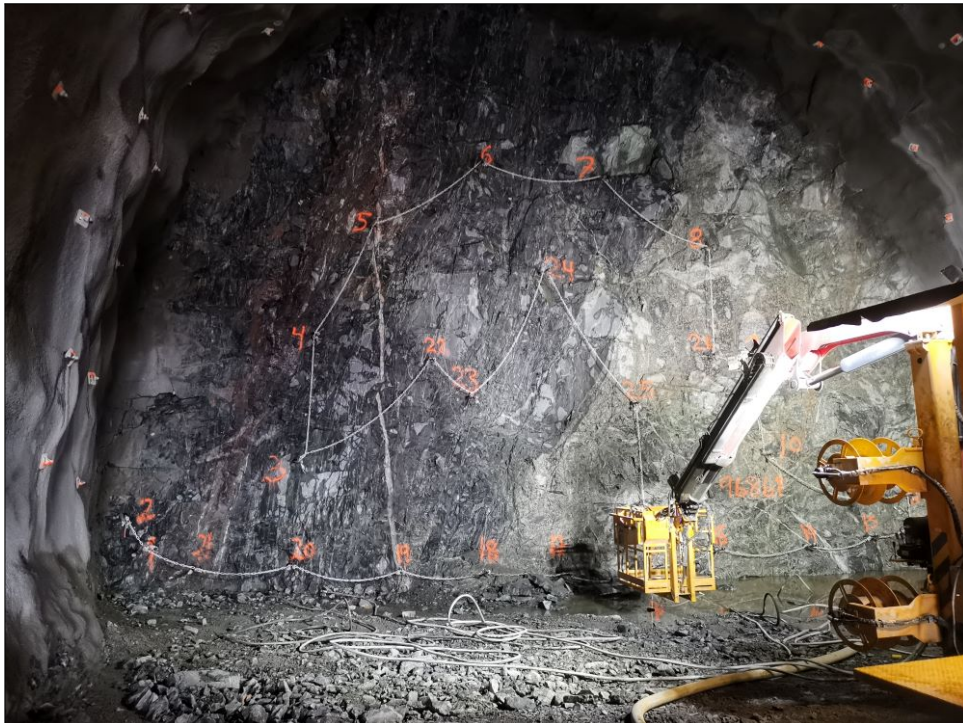
Figure 8.8: Amphibolite (left side) with a visible foliation parallel with the bedding with a strike/dip of 180/65SE. The picture was taken at Espa tunnel face.
