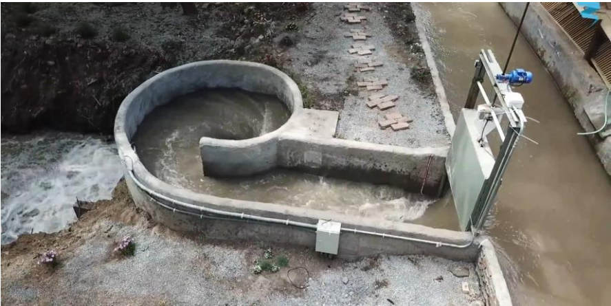
Figure 3 - An example of a whirlpool turbine and the amount of concrete and secondary structures needed for its installation. Source: (Wonderful Engineering, 2023).
