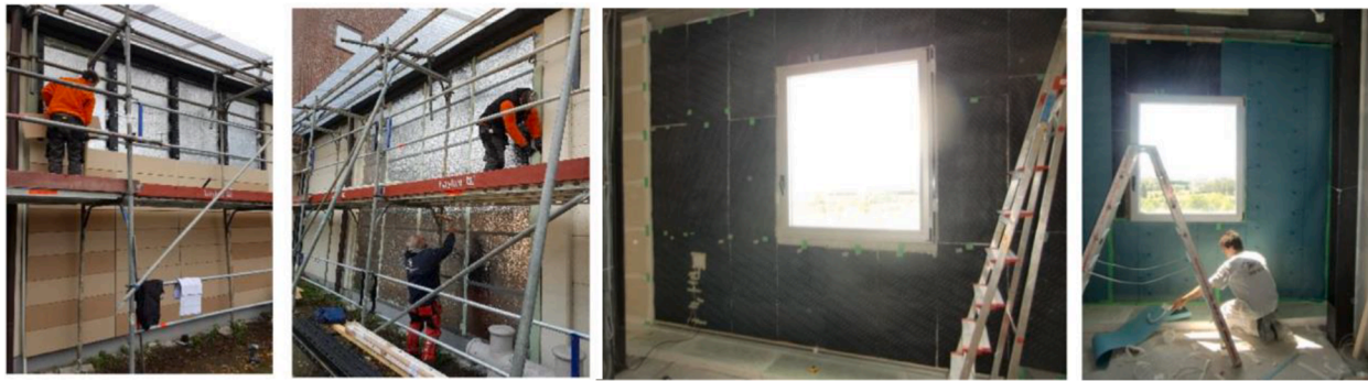
Fig. 4.2. External ventilated façade retrofitting with VIPs in Malmö (two left photos) and internal installation of VIPs in KUBIK by TecNALIA (two right photos) [116].
