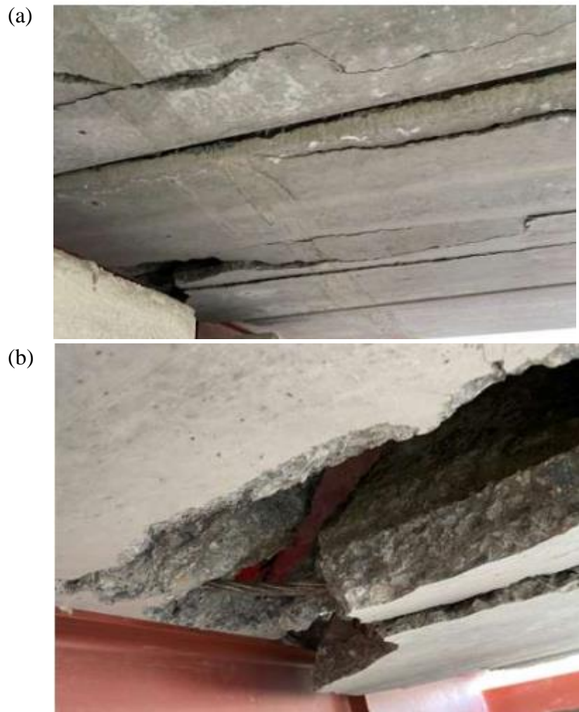
Figure 16: Floor damage (T3F2); (a) Bottom face of floor with severe damage in middle and neighbouring elements; (b) Detail showing exposed prestressing strand
