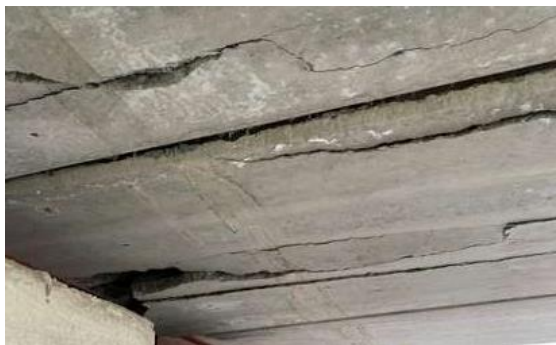
c) The area close to the support at right side after second impact
