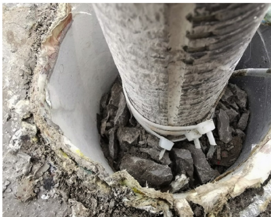
Fig. 31. Crushed grout in the borehole of anchor 3C after the endplate slid approximately 580 mm.
