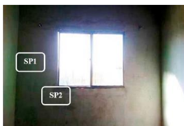
Figure 20. Location of points of dry area and area affected by humidity on the subjected wall [87].
