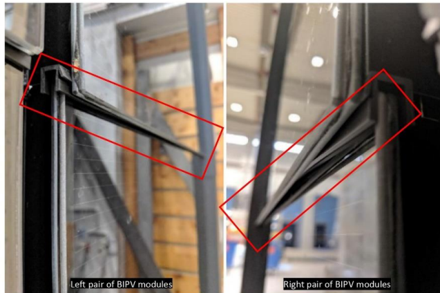
Fig. 20. The rubber profile between the pairs of BIPV modules (marked with white rectangles) inspected after wind-driven rain testing in the RAWI box for BIPV system 3 installed with steel roof plates. The rubber profile between right pair of modules was dislocated and had lost its sealing function, while the rubber profile between the left pair of modules was still in place and thus no water leaked through it.
