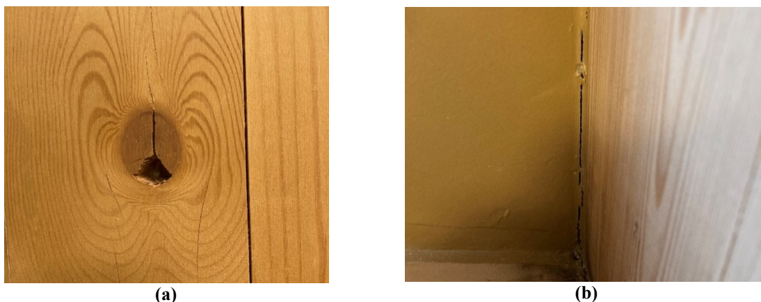
FIGURE 3. Knot hole in external CLT-element (a) and cracked sealing joint between CLT-element and external wall (b)
