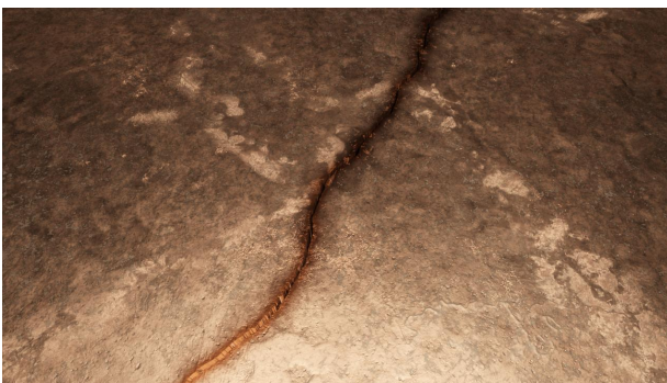
Figure 3.34.: Rendered image of a crack with a Crack Width of \simeq 5mm .
