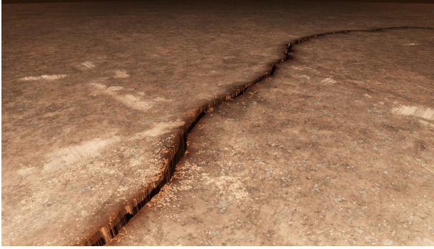
Figure 3.42.: Rendered image of a crack with a Crack Edge Height of 50\text{mm} .
