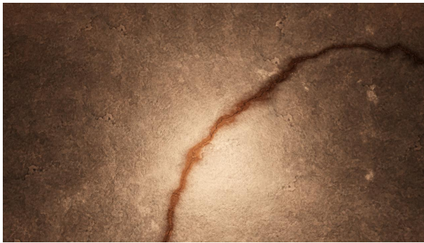
Figure 3.14.: Rendered image of a crack with a Noise Texture W of 30.
