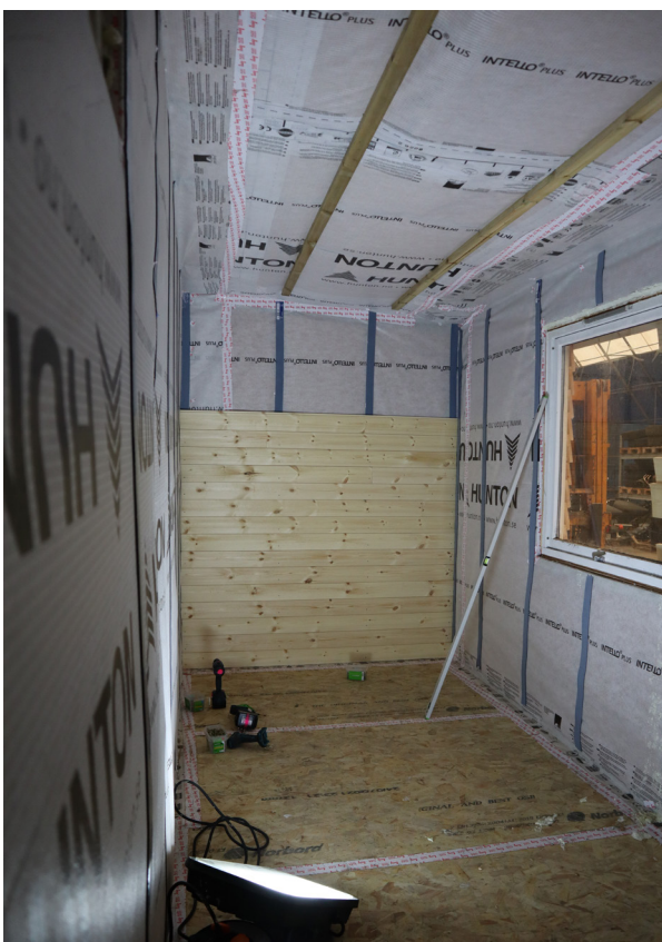
FIGURE 118. Thick tape is added to studs to protect the vapour barrier as the interior cladding is mounted
