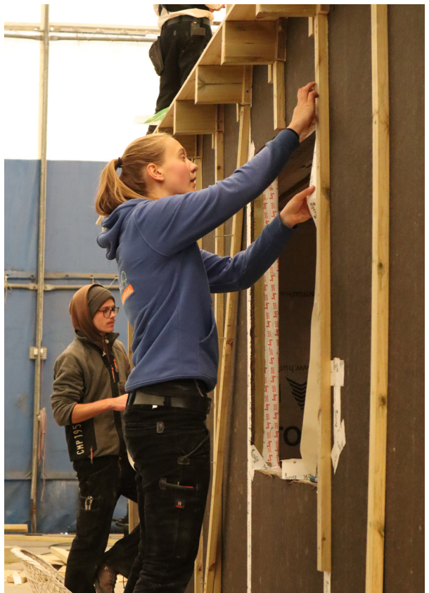
Cladding studs are added to the exterior and roof beams are installed
