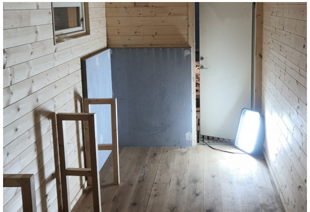
FIGURE 127. Fire-proof paneling adhered to wall in stove corner
