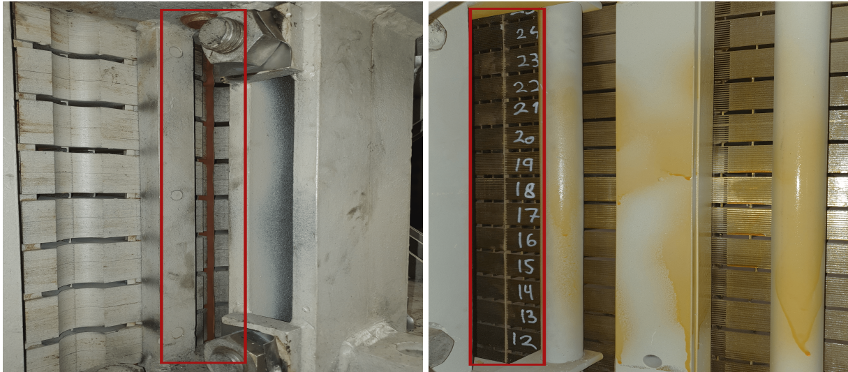
(a) Field-joint in a stator core. The paper used as insulation between the stator segments can be observed.
