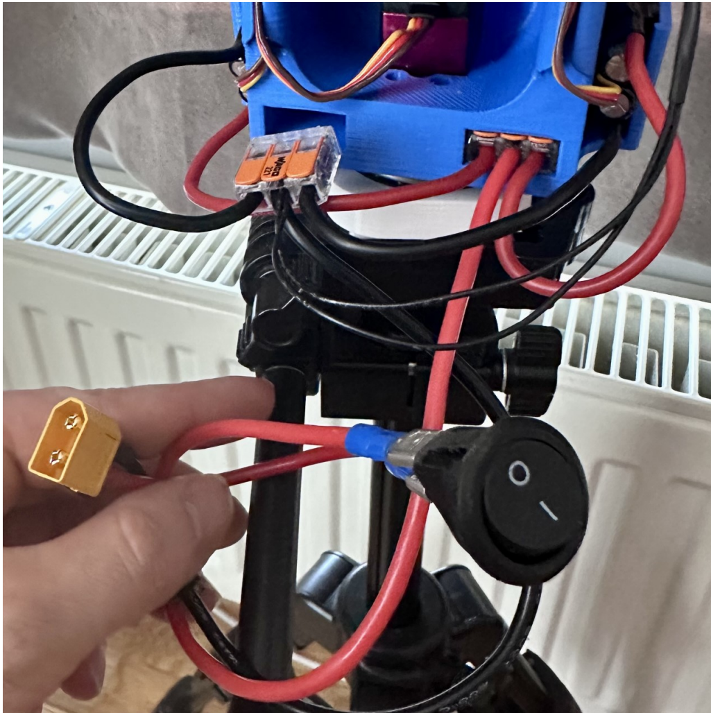
Figure 64: Connection of main current using WAGO connectors.
