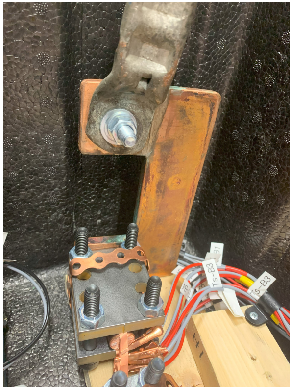
Fig. 29: Additional copper that was added to make it easier to connect the bigger dimension copper cables.
