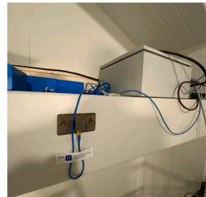
(c) Testing equipment including the control box and accelerometer mounted on the glulam beam
