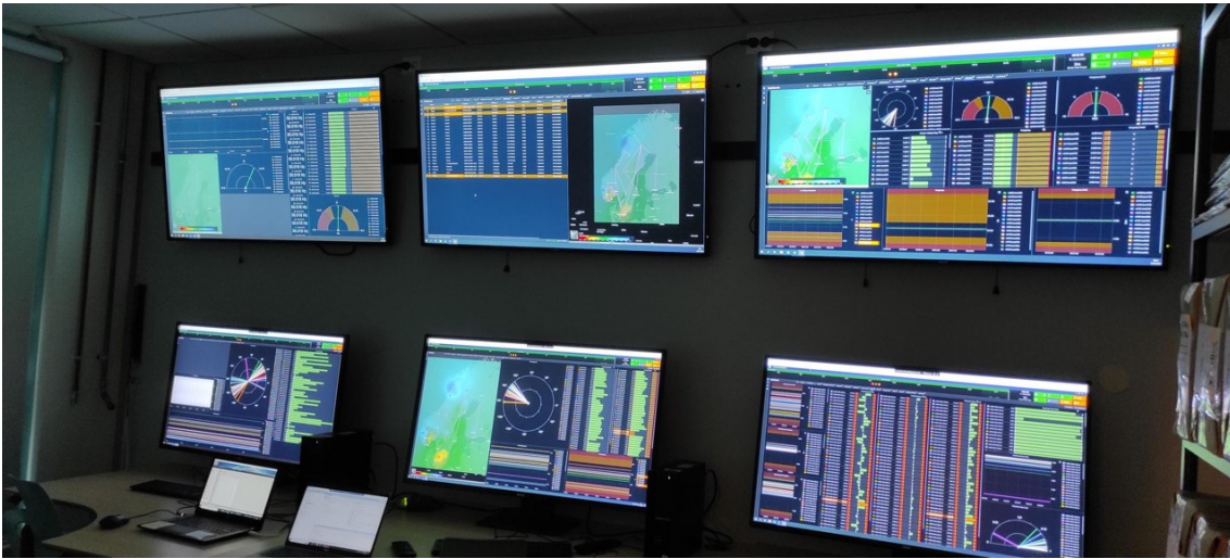
Figure 26: Picture of the control room
