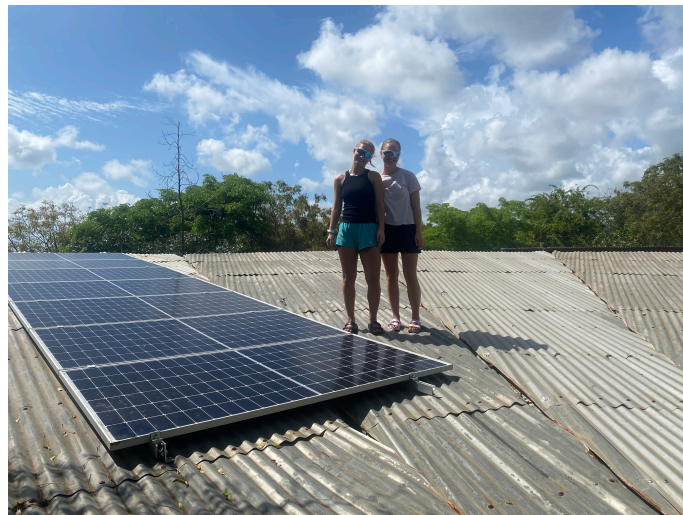
Figure 1: The PV panels of the existing system at Eco Moyo in November 2022.
