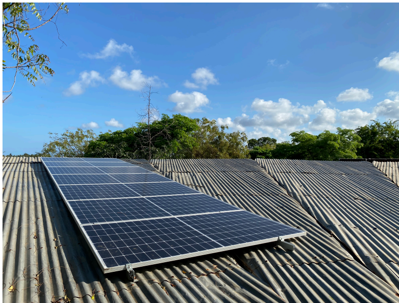
Figure 13: The PV panels located on the roof of Class 5 at Eco Moyo.
