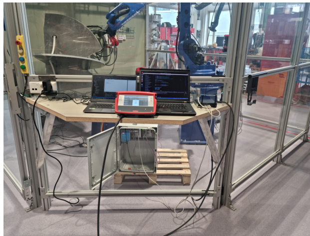
Figure 22: A image depicting the test done with a Linux computer from another angle, showing the PLC in the control cabinet.
