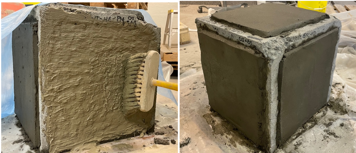
Figure 5-7: Concrete repair: Application of Rep 05 (left) and after hand application of Rep 65 (right)
