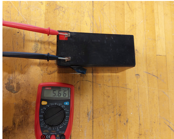
Figure 31: Measuring of batteries for logging. As shown, the voltage is way lower than the nominal 12 volts.
