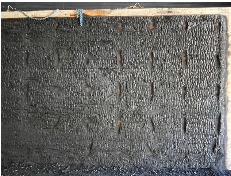
Figure 2.3 Holes in the ceiling elements from the Compartment Test, in 50 cm x 50 cm grids used for charring depth measurements.
