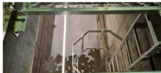
Figure 9: The sedimentation basin at the Vålerenga tunnel
