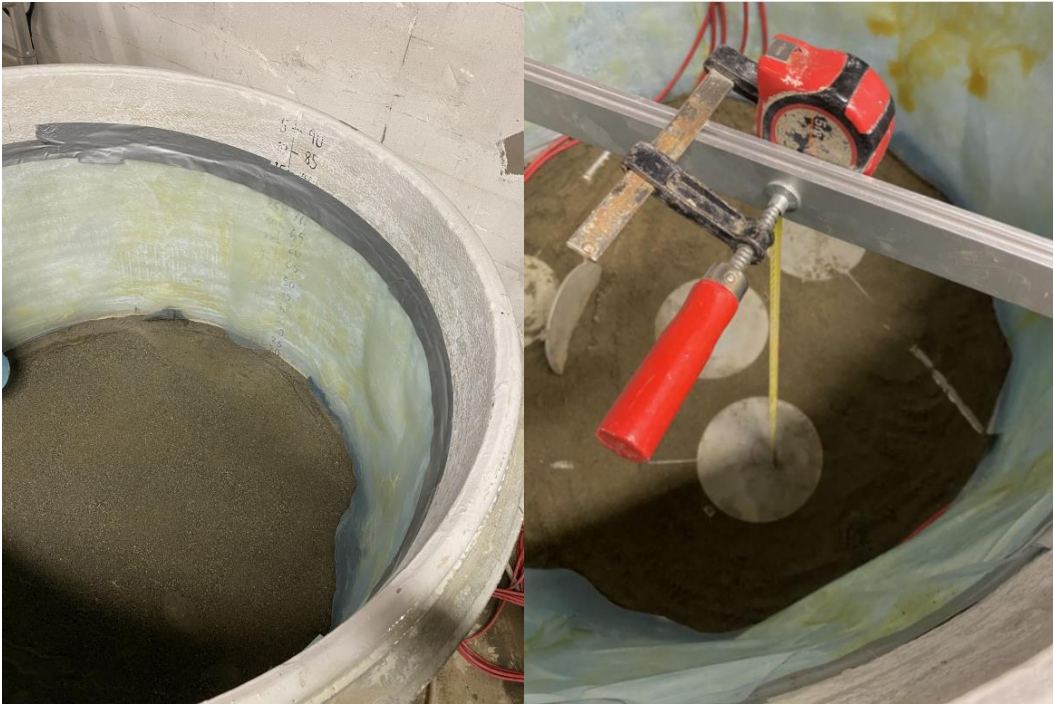
Figure 1: Added plastic lining with low-friction grease.
