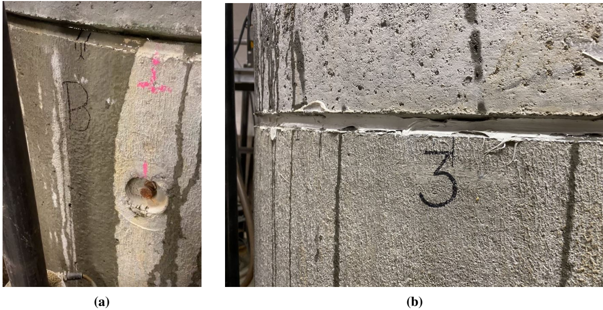
Figure 5.4: Fig 5.4a: Leaking of the chamber due to a defect in the top element. 5.4b: Leakage temporarily fixed with tec7.
