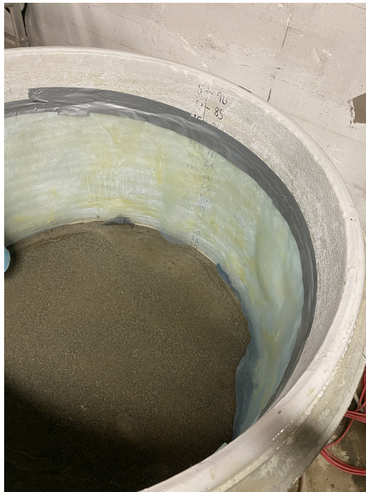
Figure 3.4: Plastic lining was inserted to work as a floating ring reducing the arching effects on the wall.
