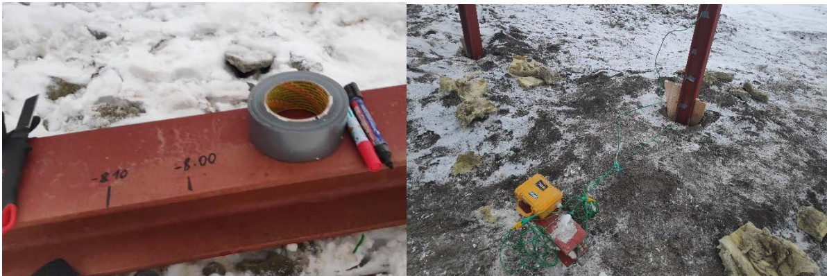
Figure A.6. Thermocouples installation 16/02/2022: (a) – showing the depth below the ground, and (b) – showing the logger (yellow) and 2 green channels going on along the pile length
