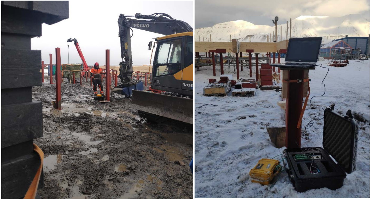
Figure A.10. Thermocouple and Thermistor installation after 16/03/2022: (a) – concrete pouring via the excavator cup on the analyzed pile located close to the existing building, and (b) – checking the setup of the thermocouple and thermistors.
