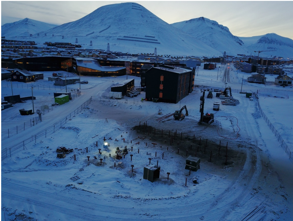
Figure A.4. Drone image from the North direction - Pile installation and the existing infrastructure is visible (picture belongs to Hæhre Arctic).
