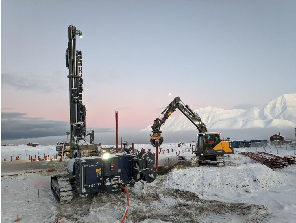
Figure A.5. Image shows the drilling machine (left) and driven pile with the crawler excavator by use of a grapple claw (right)
