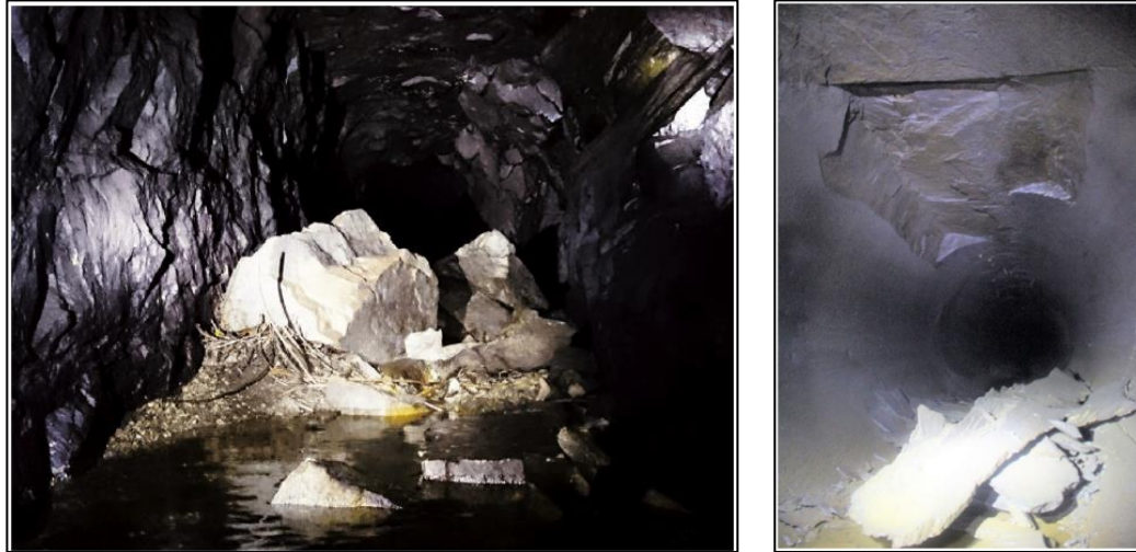
Figure 2-5: Example of rock fall which may be due to dynamic pressure from transients (left) (Bråtveit et al., 2016). Right: Block fall seen in Ulset headrace tunnel in 2017 (Neupane, Vereide, et al., 2021)
