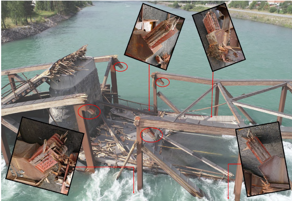
Figure 19: Red rings marks the upper nodes, while images represent the nodes that were under water. These nodes connected the diagonals in the main span (Statens havarikommisjon 2022b).
