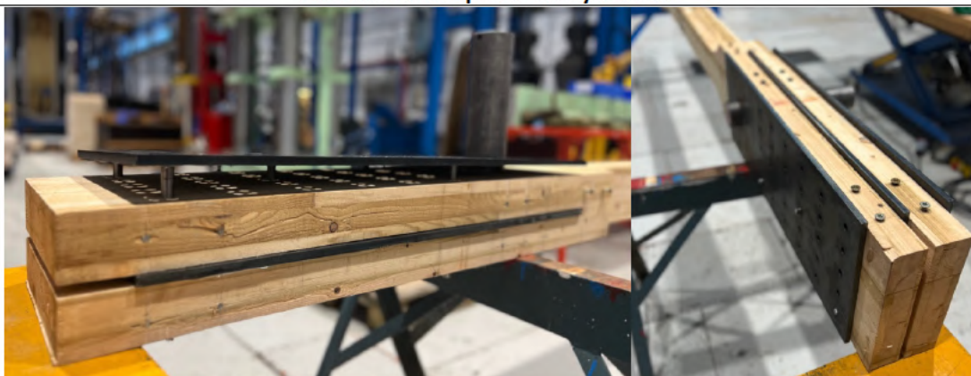
Crooked holes in S3 posed challenges for plate alignment, requiring pre-drilled dowel holes
