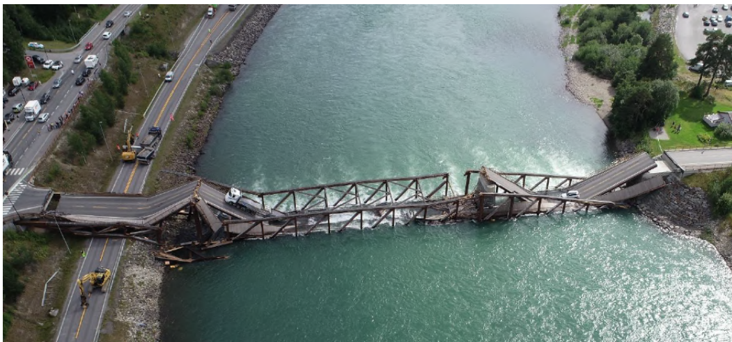
Figure 18: A truck with a trailer and a car were on the bridge at the time of the collapse (Statens havarikommisjon 2022a).
