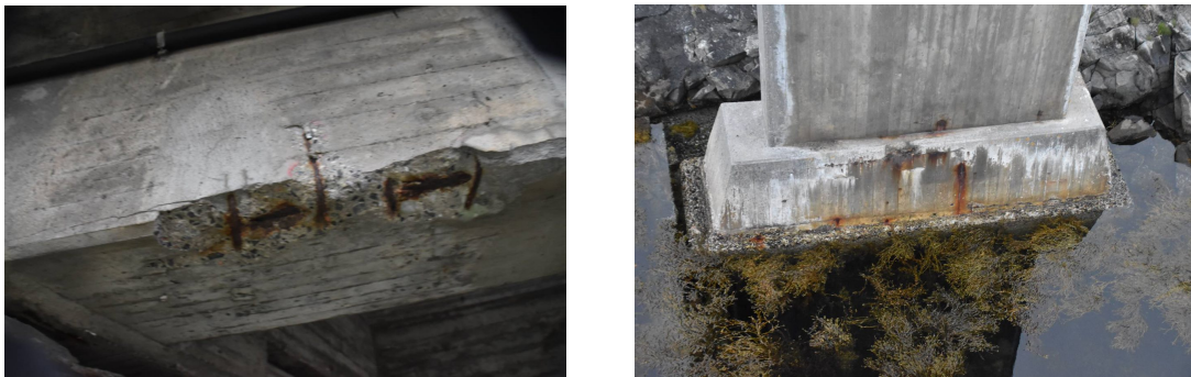
Figure 16: Pictures of peeling and rust colouring on Herøysund Bridge from Brutus.
