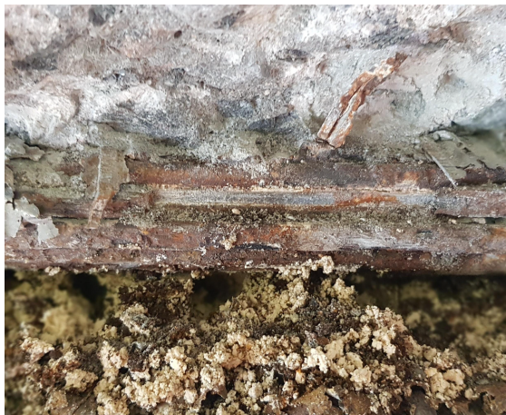
(b) Wires with no bond to the concrete on the bottom side
