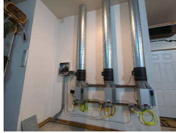
Figure 5: ASIC in technical room with heat transportation through ductwork.
