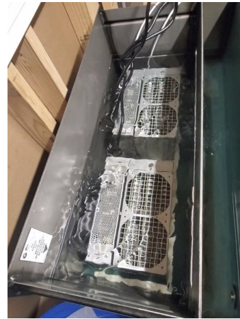
Figure 6: ASIC in technical room with waterborne heat transportation.
