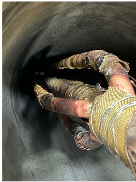
Figure 8.15: Inside the collector with new modifications.
