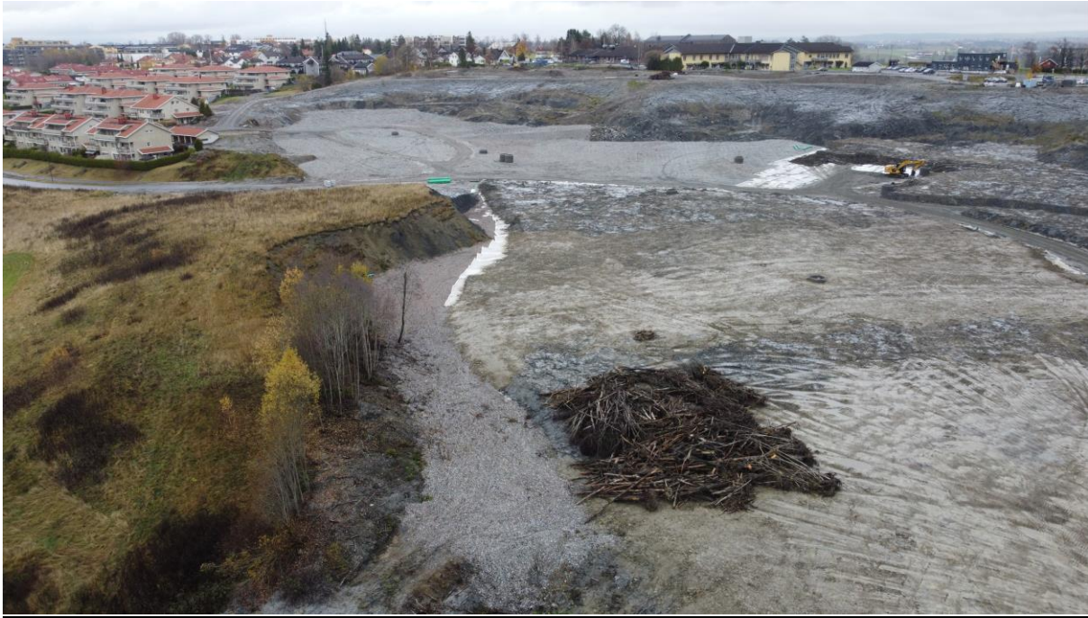
Figure 17. Inspection 27.10.22. Clay is filled on top of the layer of gravel. Photocredit: NGI
