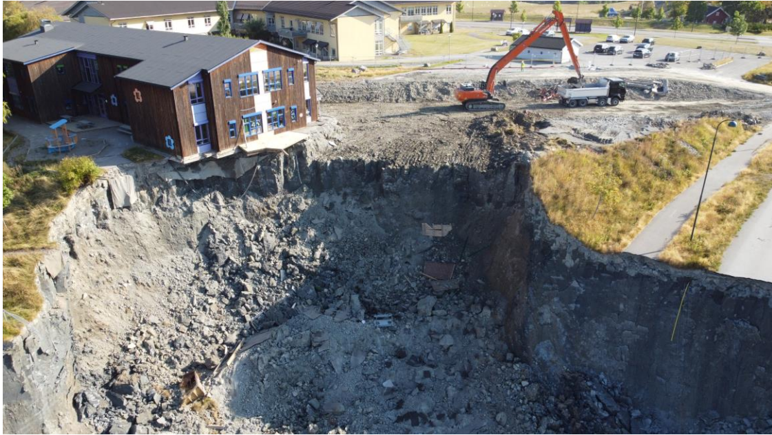
Figure 13. Dronephoto 02.09.21. Excavator at work relieving masses behind the kindergarden. Photocredit: Gjerdrum kommune.
