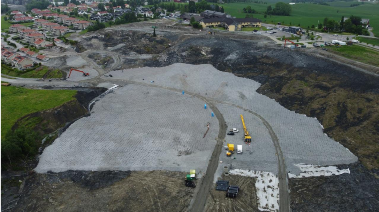
Figure 15. Dronephoto 10.06.22. Vertical drainage installed for most of the area south of Fjellinna. Photocredit: Gjerdrum kommune
