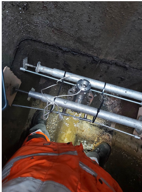
Figure 3.17: The camera was mounted in the manhole by sliding it into a metal holster resting on two expandable horizontal bars spanning between the manhole walls.
