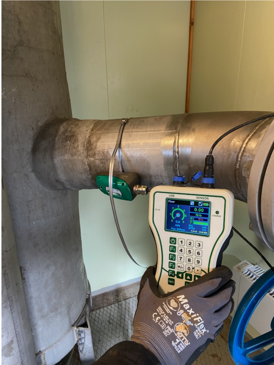
Figure 4.4: A Mounted FlowPulse Ultrasonic Clamp-on Flow Sensor with the Handheld Controller, Used for Measuring the Sewage Flow Rates.
