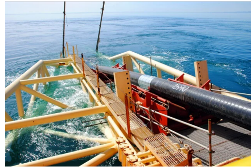
(b) Offshore pipes
