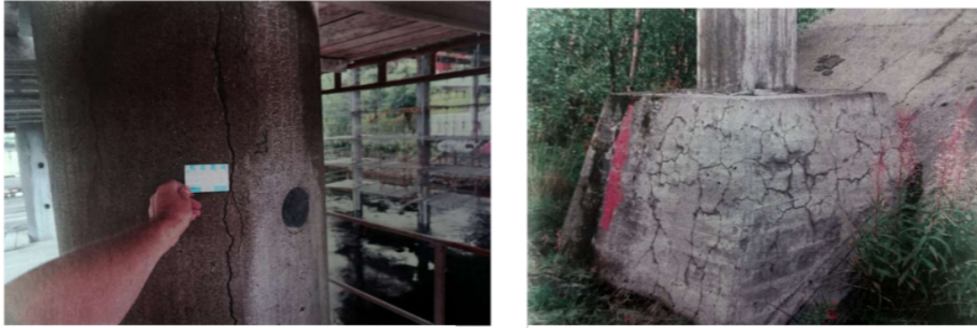
Figure 4.7: Typical crack pattern in column and foundation due to ASR [21]
