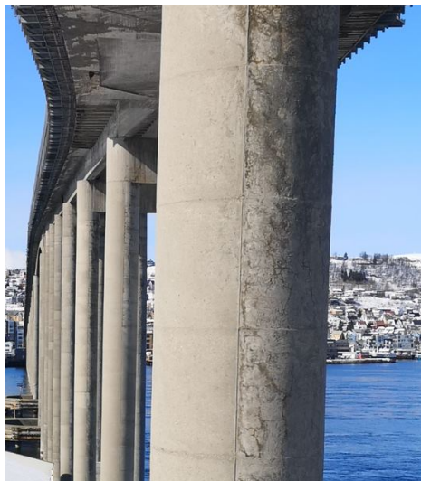
Figure 5.1: Difference between ASR on the south and north side of the column of the Tromsø Bridge
